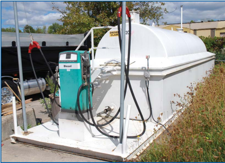
DIESEL STORAGE TANK
